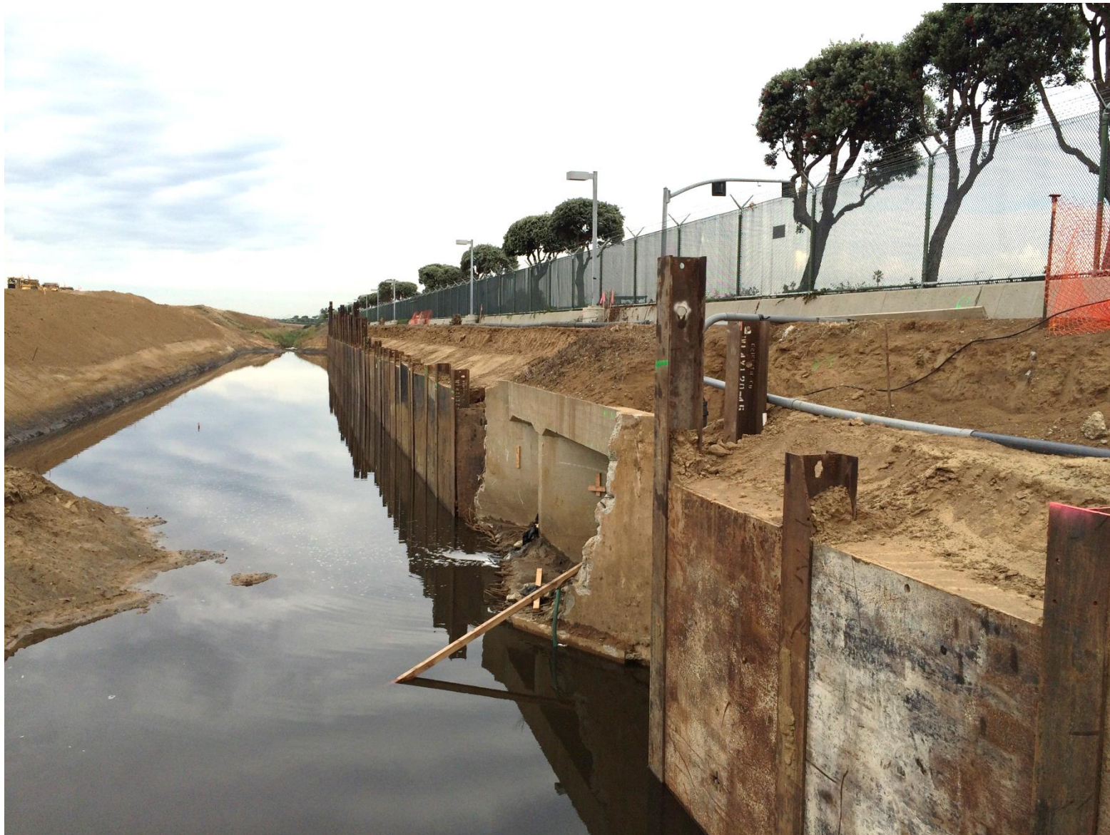
Argo Ditch after July rain. Lincoln Blvd outlet on the right. – 7/20/15
