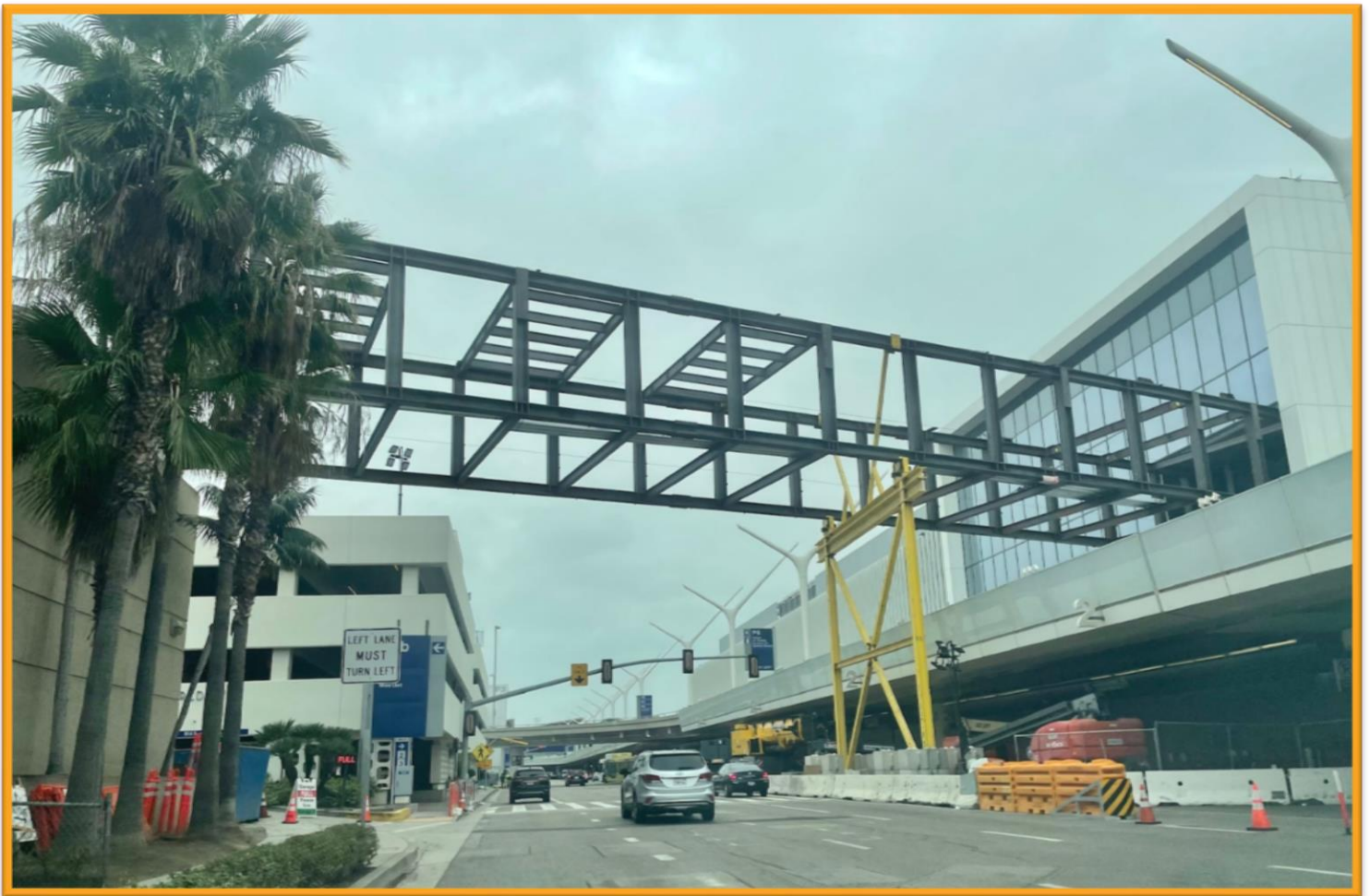
Structural components of the T2.5 Pedestrian Bridge have been installed over both level roadways
